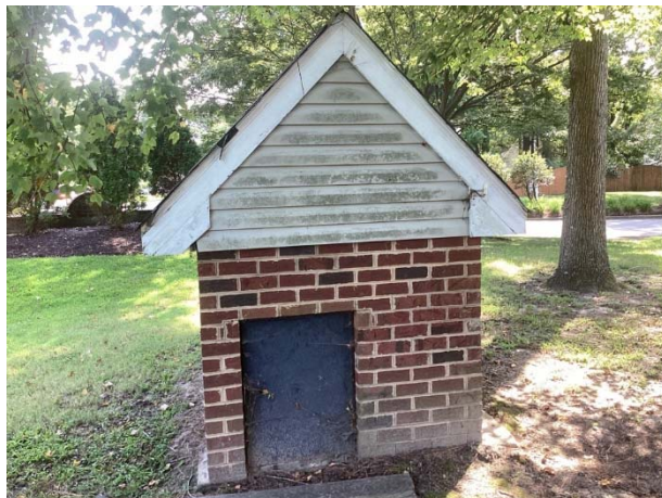
Pump house overview- Note trim deterioration
