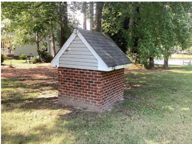
Pump house overview
